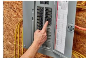
Figure 1 Electrical panel image. Source: How to Install a 240-Volt Circuit Breaker (thespruce.com)
